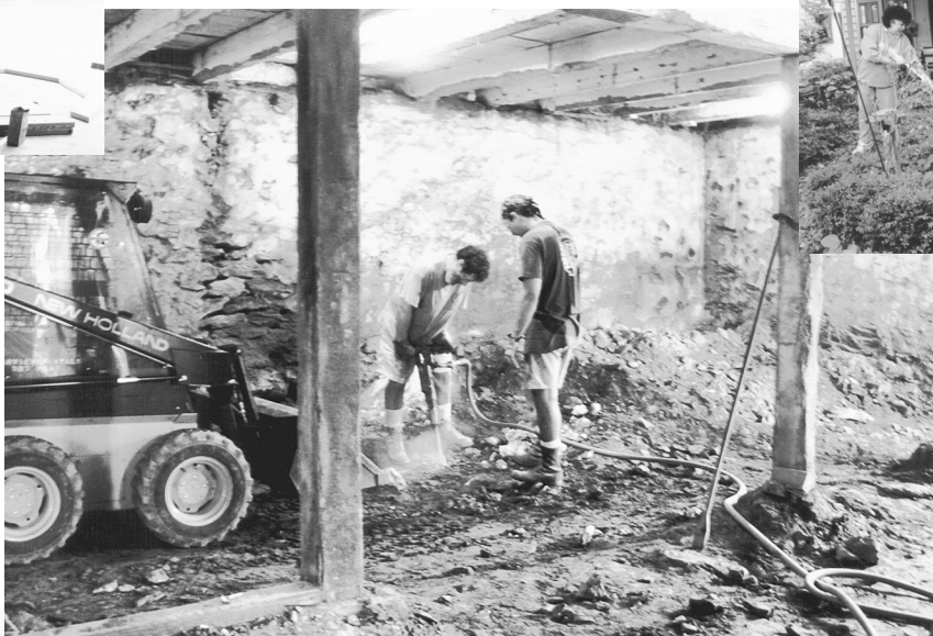
▽ Parent Tom Strauss and a community service volunteer hammer through the barn's rock foundation to prepare for heated work areas, offices, kitchen, shower, and wheelchair-accessible restrooms.
